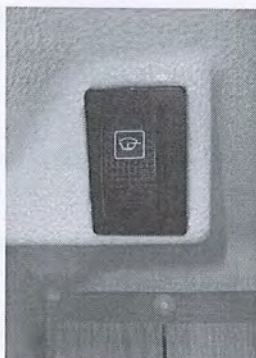
Shower pump switch
