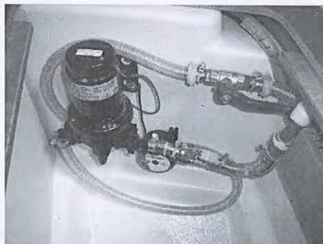
Fresh water pump
