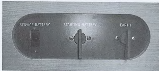
Main switch panel
